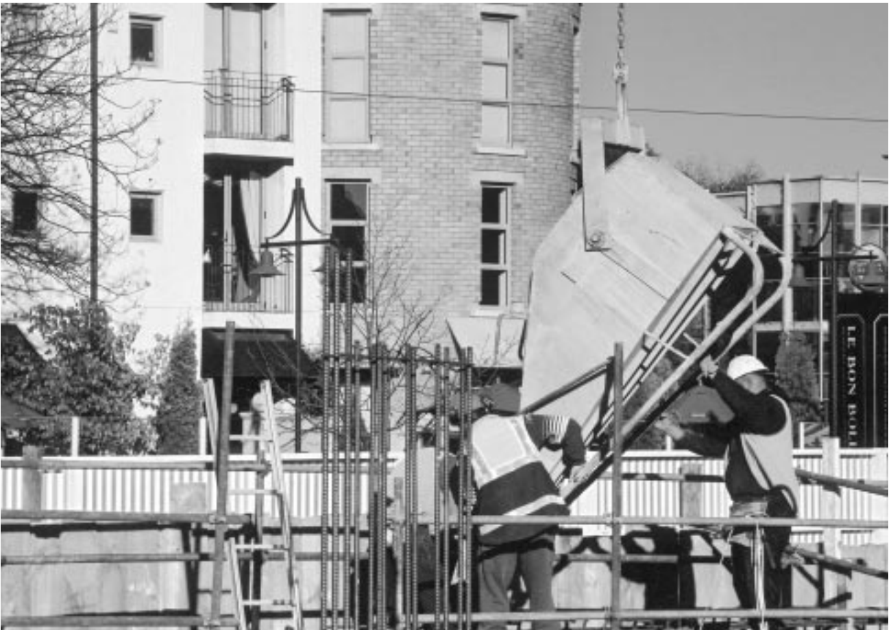
Construction workers guide a concrete skip, which has been swung into place by the overhead tower crane, before pouring starts along the Worcester Boulevard perimeter.
