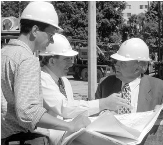
Andrew Macgregor, Mark Noonan (Council's Project Co-ordinator) and Cr Wright check plans on site - now a "hard hat area."
