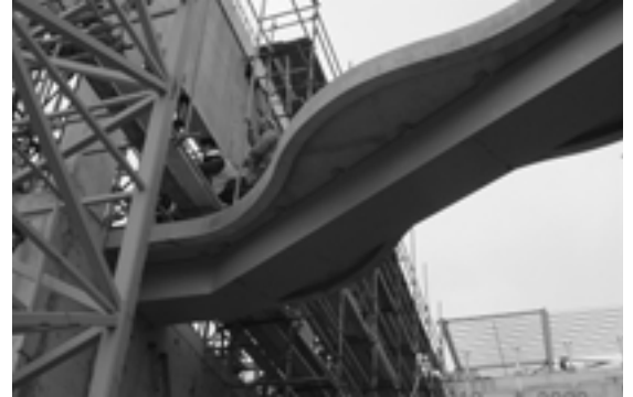
Construction workers at one end of the wavy bridge. The bridge is one of the key areas of work during autumn.
